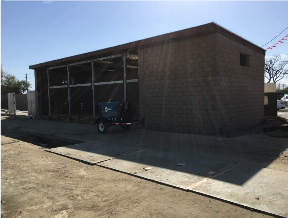
Electrical Building Construction Zone
