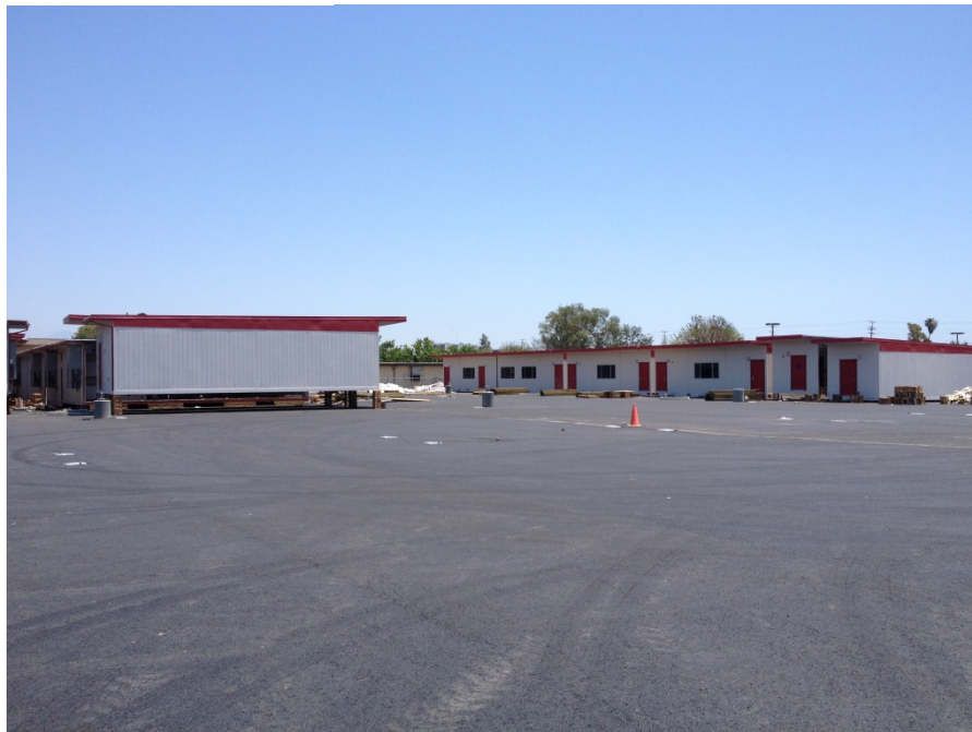
Portable Village modular buildings in process of being set on sleeper foundations.
